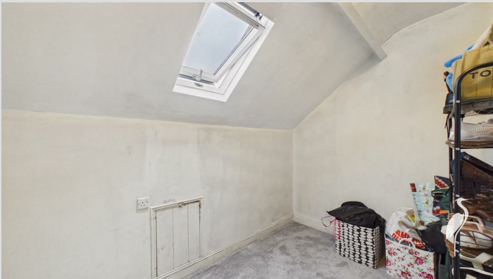
Double glazed skylight window.
